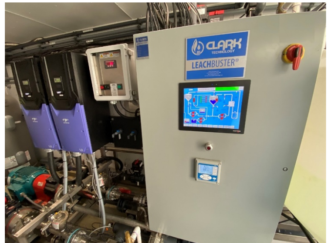
Photograph 2: Standard interior view of the control panel, pumps, VFDs, and other equipment for a typical Containerized WWTP. Virginia CLB is shown.
