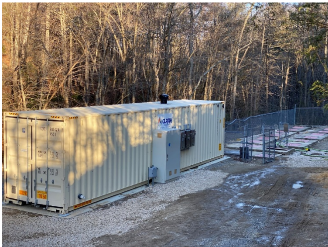
Photograph 1: Typical Containerized WWTP installation. Virginia CLB is shown.
